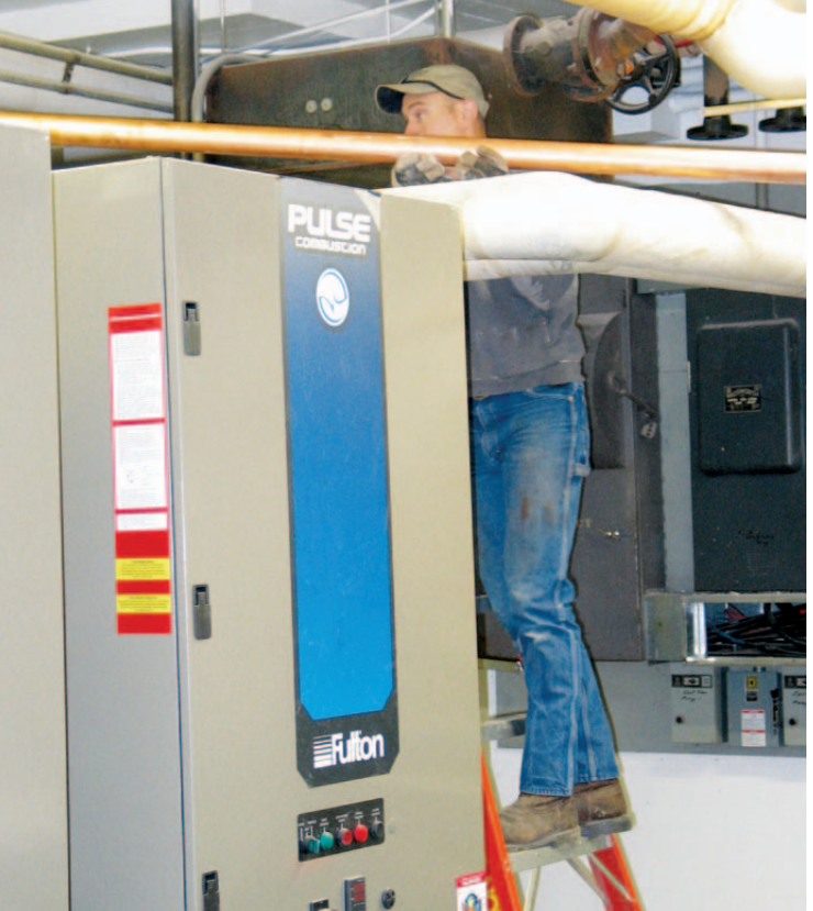
Plumbers & Steamfitters 11's Drew Smykalski, employed by A.W. Kuettel, guides copper piping over one of two new boilers being installed in the Labor Temple.
